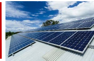
Solar Roof top
